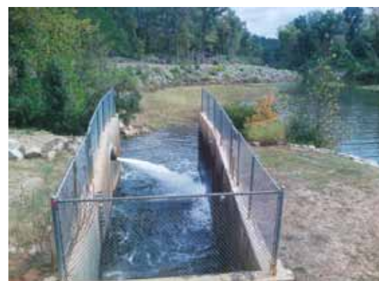
Douglas County now diverts 6 million gallons of reclaimed wastewater daily from a treatment plant to augment Dog River flows.
