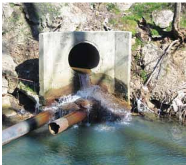
Treated drinking water flowed from a storm drain under Ansley Mall into Clear Creek; this leak was stopped in May.
