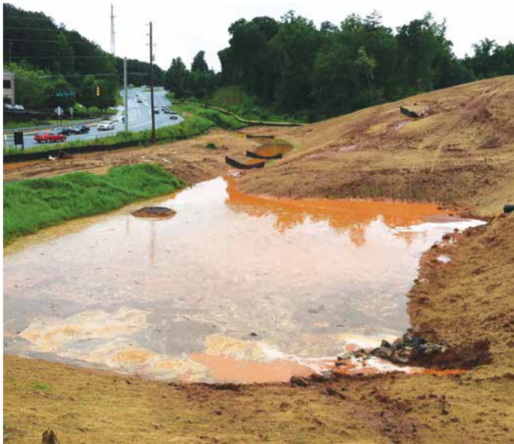
Without the proper erosion and sediment control measures installed during construction, downstream waterways fill with mud, resulting in environmental and economic damage.
