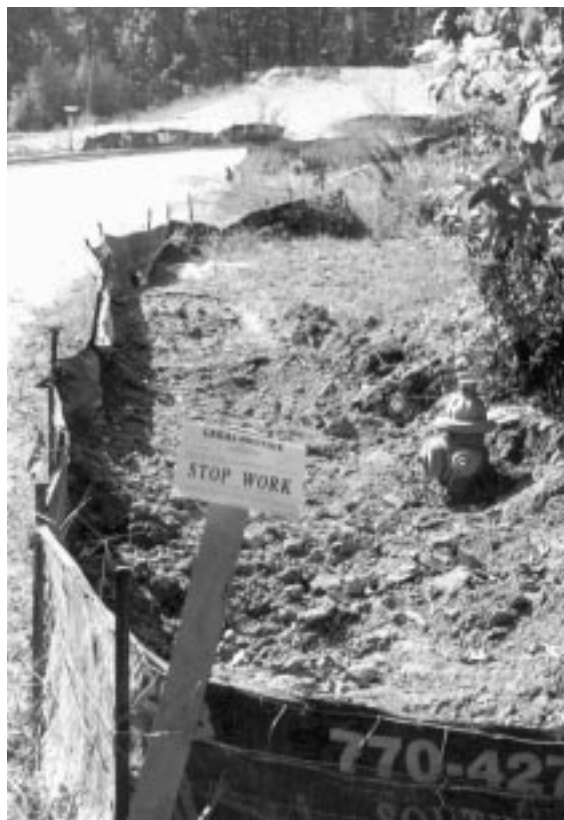
Silt fence with "STOP WORK": Inspectors have a new "tool"- MANDATORY Stop Works were added to the list of most recent erosion changes.
