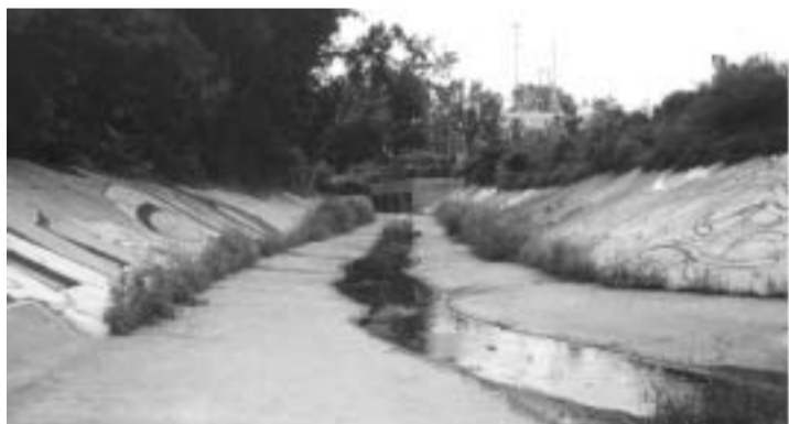
No natural buffer along Clear Creek below Atlanta's Combined Sewer Overflow facility.
