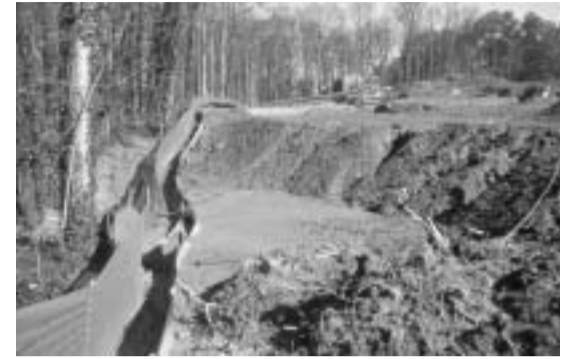
Dirt runs off construction site due to insufficient Best Management Practices (BMPs).
